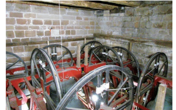
The new steel frame with bells and wheels and the C17th wooden frame still in its original place above.
